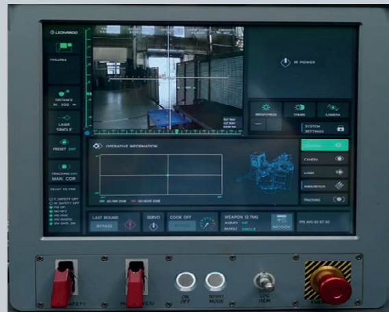
Local Control Panel
